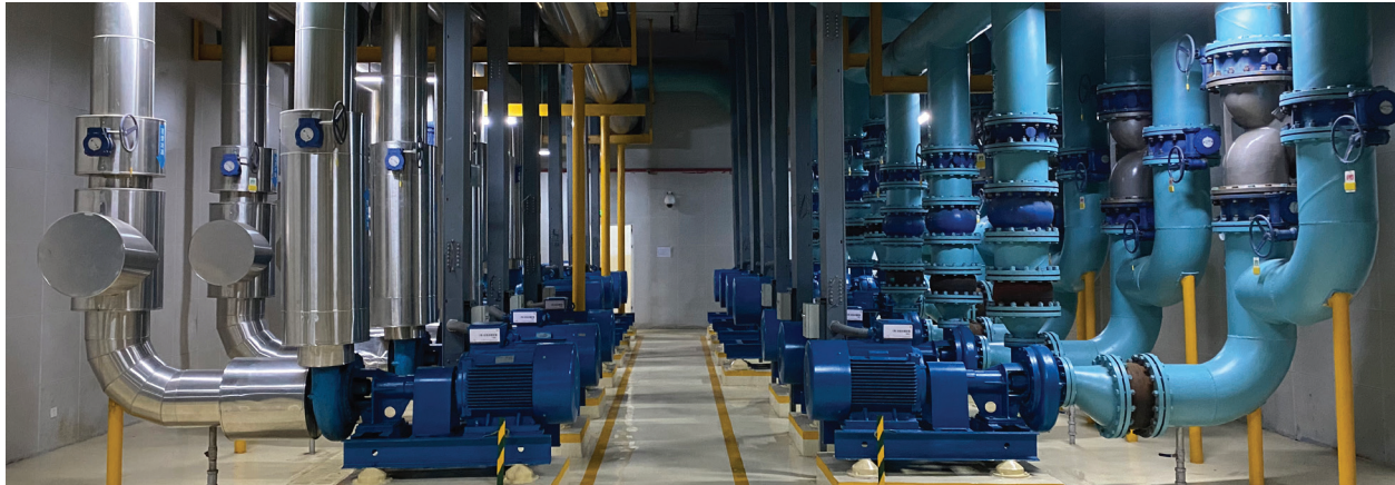
Chiller pump room in City Center Mall, Central China.
